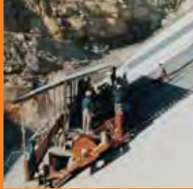
Client: Daewoo Corporation Project: Houay Ho Hydro Project, Loas. A dragscreed was designed by RMD Kwikform for placing and finishing the concrete on a 300m wide dam.
