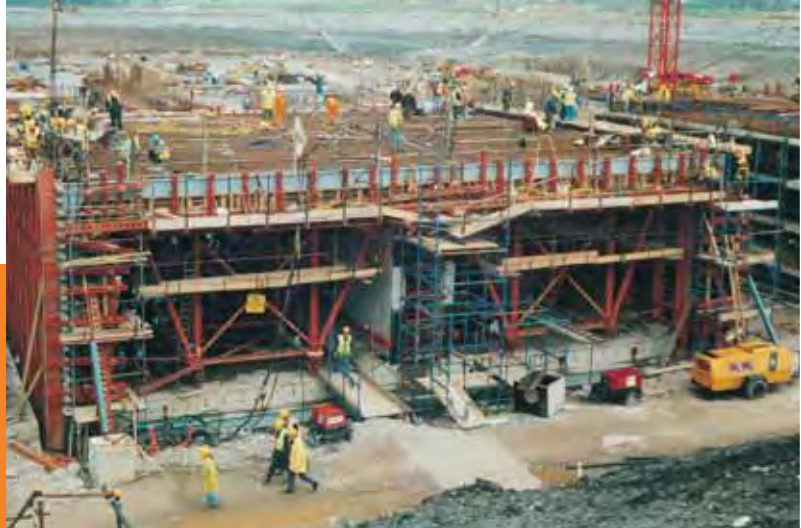
Client: Tarmac Walls JV. Project: River Lee Tunnel, Cork, Ireland. The outer walls and roof of the 610m long tunnel were cast together in a single operation using a special traveller that could be struck and re-erected rapidly.
