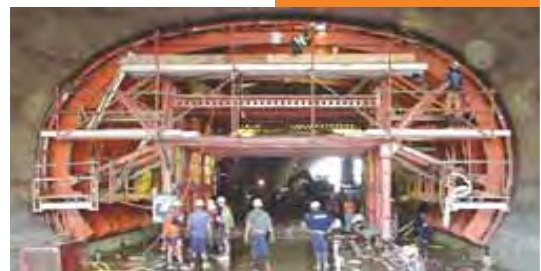
Client: Chung Soo Construction Co. Project: Nam Hai Bridge Piers, South Korea. Bull nose pier jump forms for multiple lift pier construction.
