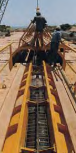
Project: Beenyup Sewage Outfall, Western Australia for the Western Australia Water Authority
