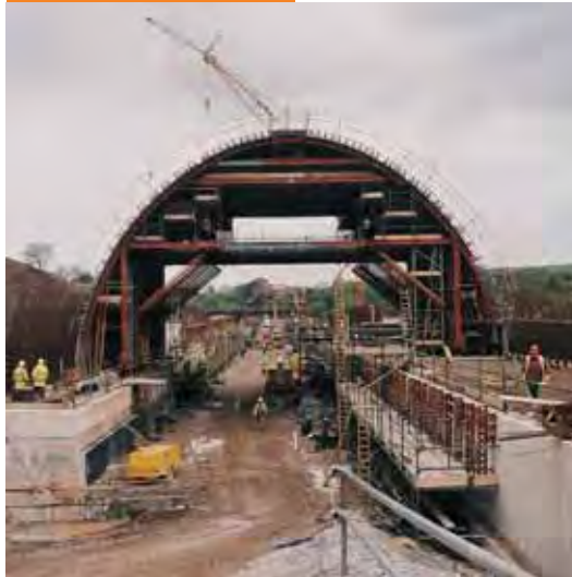
Client: Amec-Tarmac JV Project: River Bollin Tunnel Manchester Airport, UK Megashor portal frames mounted on skates either side of the tunnel. After each concrete pour, the formwork was hydraulically lowered and repositioned further down the tunnel, ready for the next pour.
