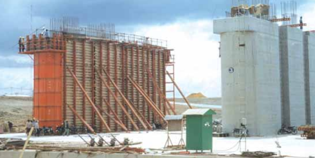
Client: China Water and Electric Project: Pak Phanang Dam Thailand. Unique design of special steel faced and standard ply faced formwork for the construction of massive reinforced dam gates.
