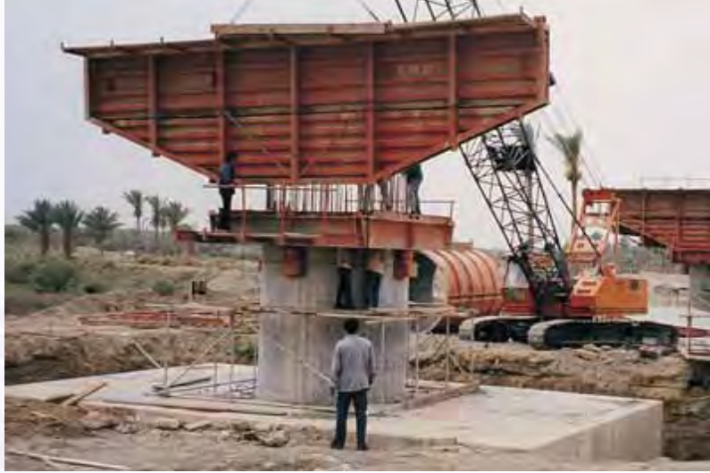
Client: Chung Soo Construction Co. Project: Nam Hai Bridge Piers, South Korea.
